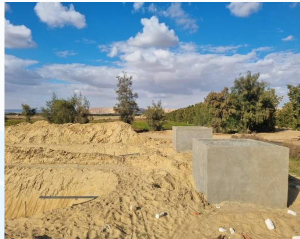
Figure 11. Constructing two overland (up-stream) tanks and two underground (down-stream) tanks. The CWT site is next to the main septic tanks of the Sekem farm El-Wahat
