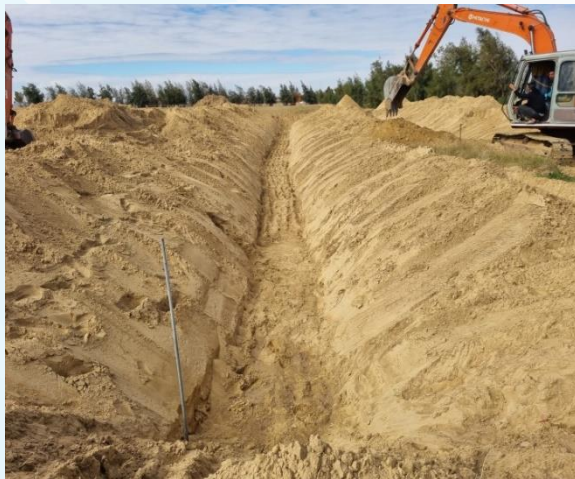
Figure 10. Configuring the trapezoidal cross section and longitudinal slope of the treatment cell. The construction of the water tanks
