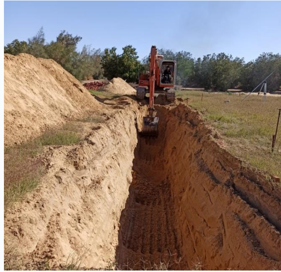
Figure 9. Excavation work of the site of the CWT pilot in Sekem El-Wahat farm, Egypt
